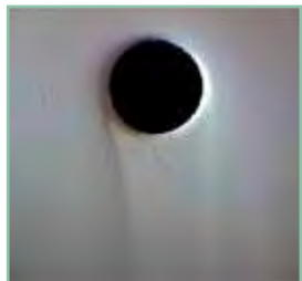
Strong sagging of paint
