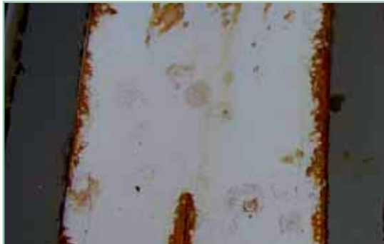
Weak corrosion protection in 2 layer system
